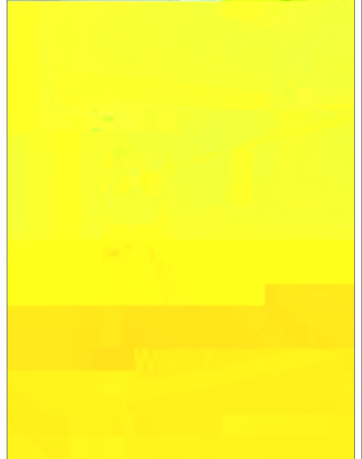
East wing corridor looking east, displayed during painting process with clearstory covered in plastic as well as classroom relights.
